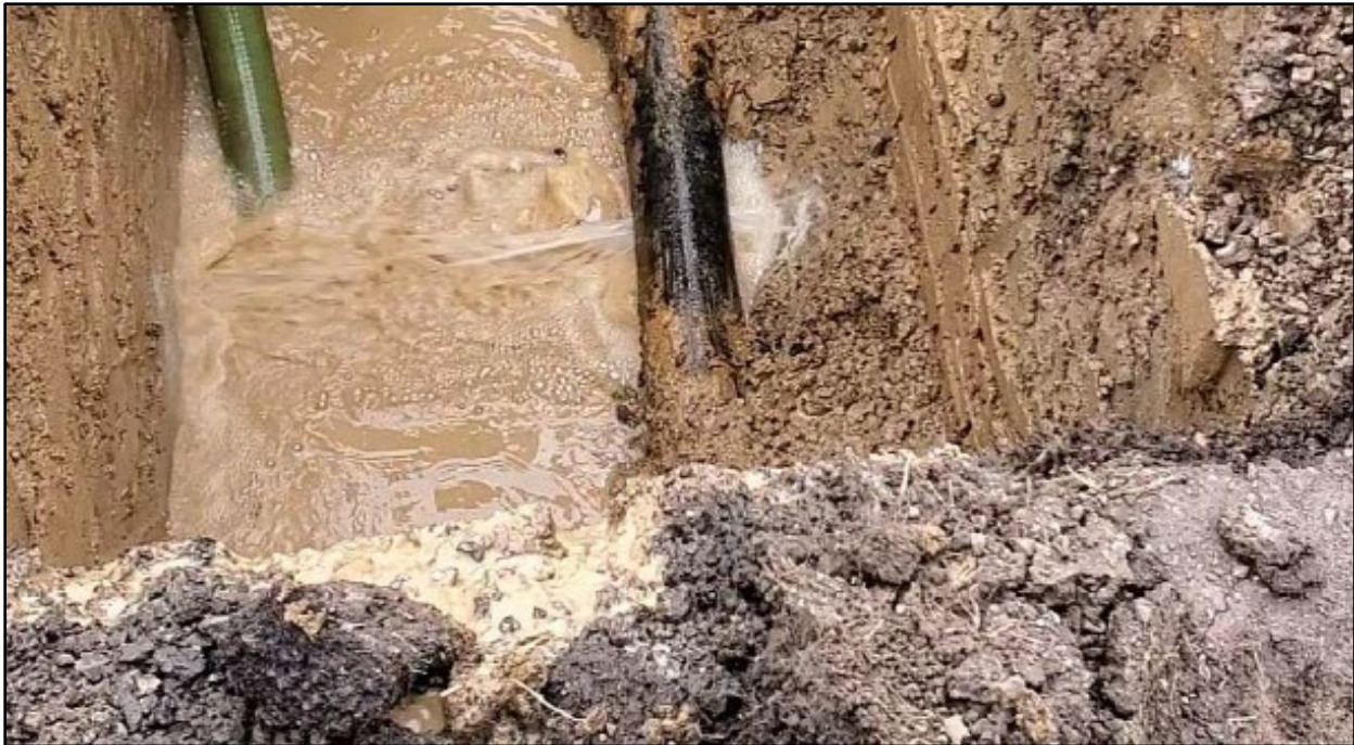
Figure 2. Photo taken during repair of a 2020 water line break along Farmer Street
